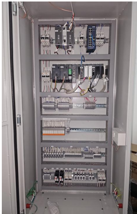
Figure 38 Programmable Automation Controllers – Microgrid and BMS (internal components view)
