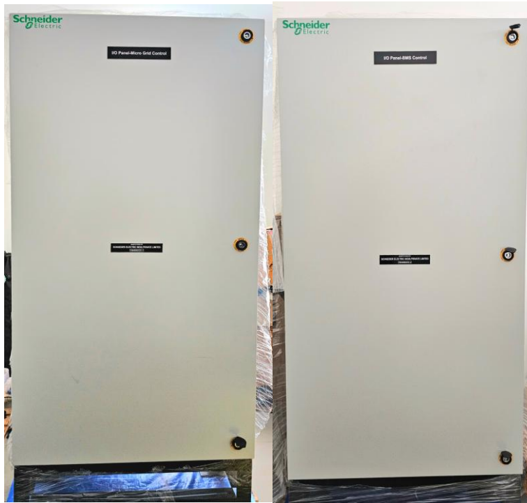
Figure 37 Programmable Automation Controllers – Microgrid and BMS (external view)
