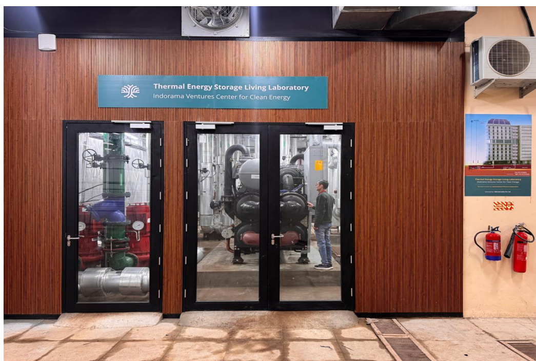
Figure 40 Thermal Energy Storage Lab
