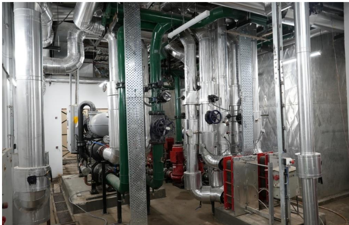
Figure 18 Thermal storage plant piping network
