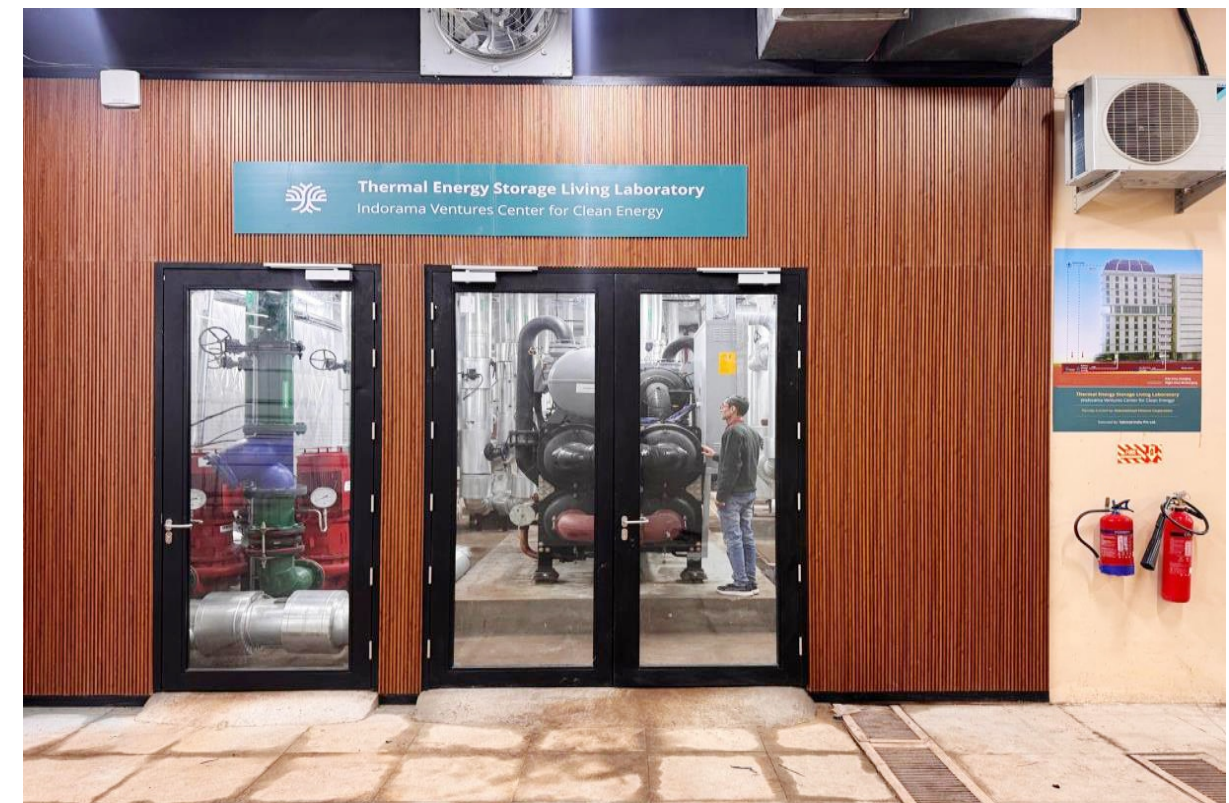
Figure 25 Thermal Energy Storage Lab
