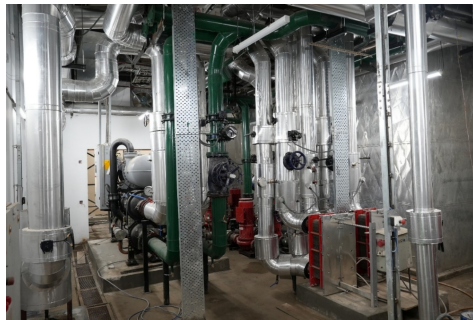
Thermal storage plant piping network
